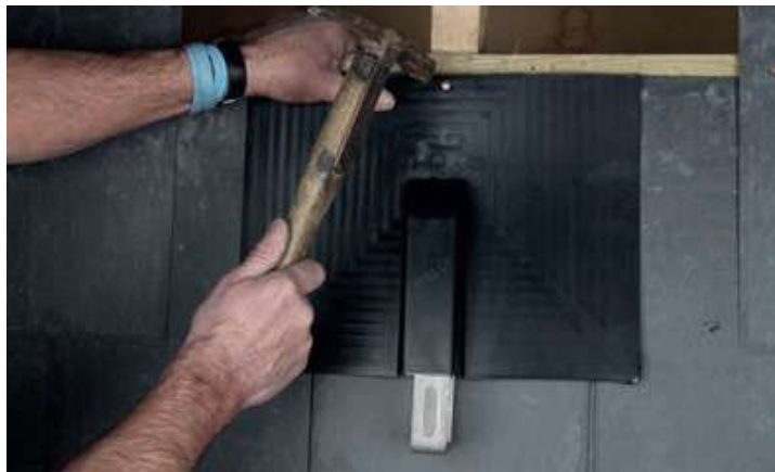
Step 3: SolarFlash can be trimmed or nailed through. If nailing through, ensure relevant line for slate size centres on the batten. Apply pressure to hold SolarFlash solid when nailing through.
